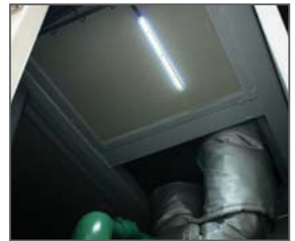
4 Internal LED lighting Eclairage interne à LED
